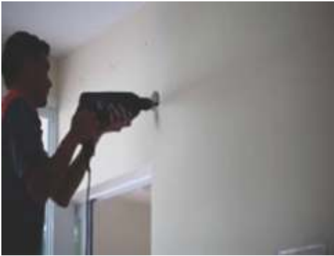
Fig 6: A simple job like drilling hole on a wall can be the reason for emergency
